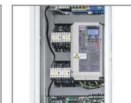
Controller MRL lift plant
