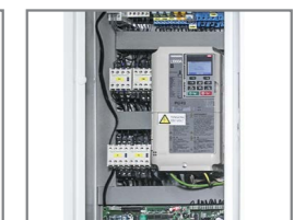
Controller MRL lift plant
